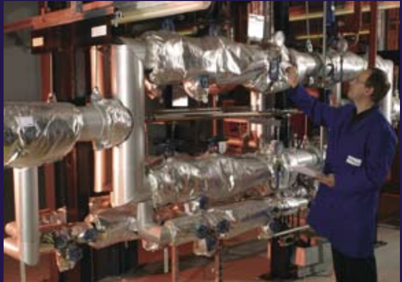
Ready assembled control systems
